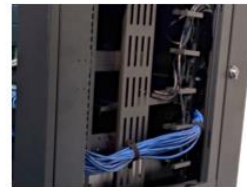
High Density Cable Management
