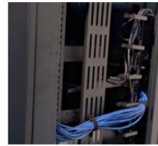
High Density Cable Management
