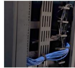
High Density Cable Management
