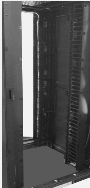
Vertical Cable Management
