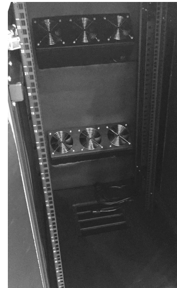
Max Load Rating and Fan Capacity
