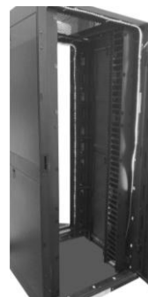
Vertical Cable Management
