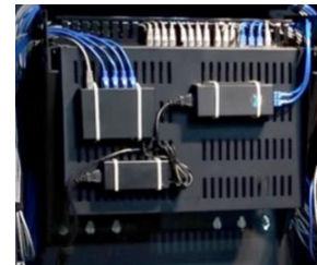
Equipment Shelving for non-EIA Mounted Equipment
